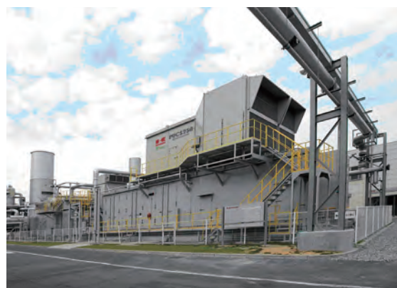
Fig. 5 Akashi Works Energy Center
