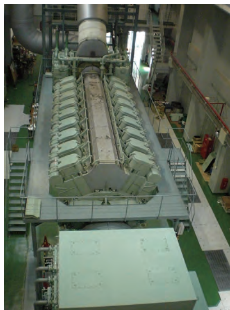
Fig. 6 Diesel generator set destined for the Okinawa Electric Power Company
