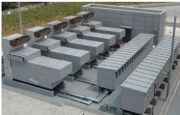
Fig. 1 3,500 kVA standby gas turbine generator set for data processing center
