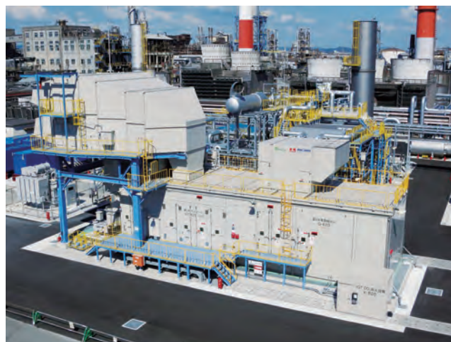
Fig. 8 Panoramic view of L30A package PUC300D and CHP plant
