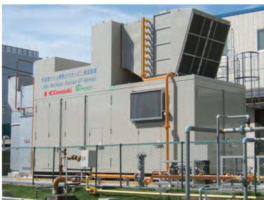
Fig. 5 Lean methane-fueled gas turbine generator set
