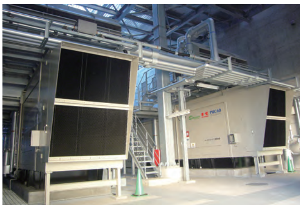
Fig. 1 Appearance of CHP unit
