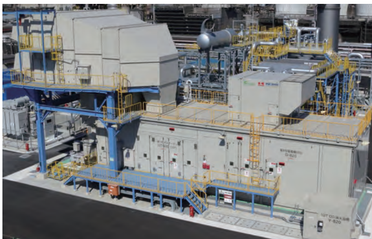
Fig. 3 30 MW class PUC300 cogeneration facility
