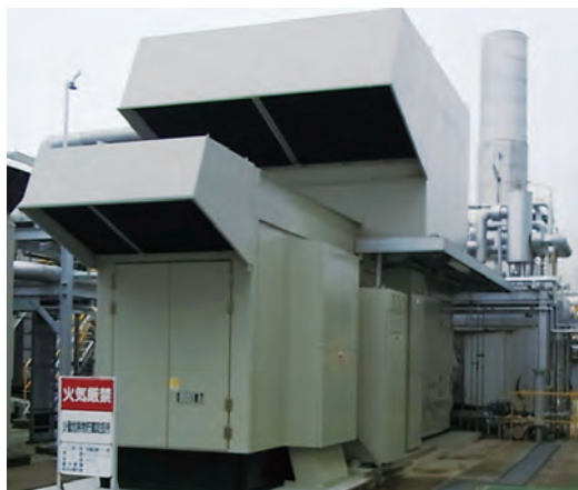
Fig. 12 Power generation plant (PUC80D) with M7A-03
