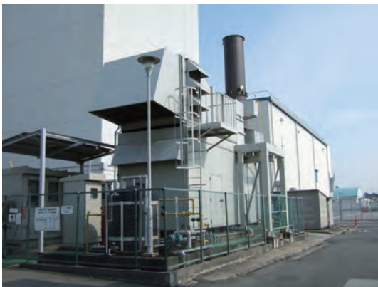
Fig. 9 Electric power plant at Akashi Works
