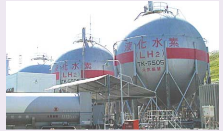
Liquid hydrogen storage-supply station for Japan's H-II rockets
