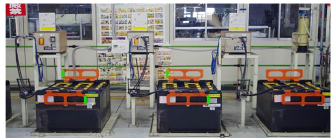
Fig. 4-2 Battery Charging Station
