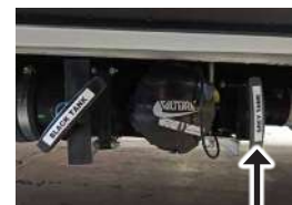
Gray Water Tank Valve
