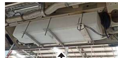
Fresh Water Tank
