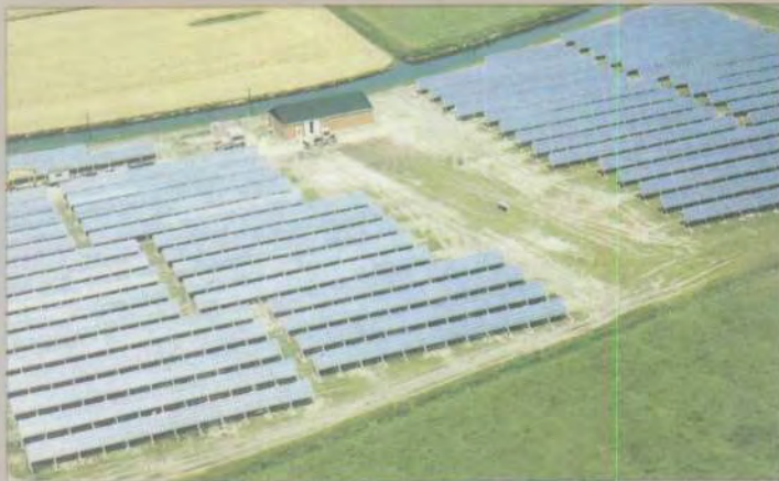
AEG solar plant on the Northsea island of Pellworm delivers a maximum of 300 kilowatt of energy.
