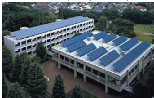
Photo 2 Photovoltaic power generation system
