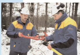
After the snowstorms at the beginning of the year, extensive work was conducted by all members of Vattenfall's network organisation.
