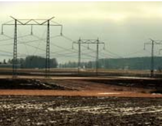
400 kW overhead power lines at Närkes-Kil.
