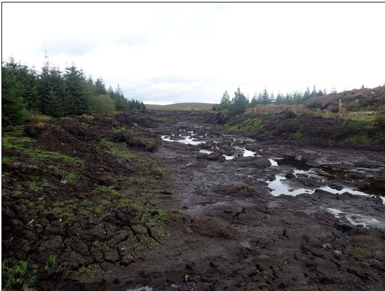
The peat slide up-gradient of the Dawn of Hope Bridge at Greaghmagh.
