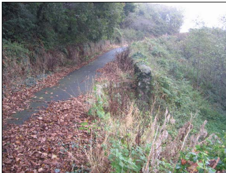
Small roadside collapse below Dunhill Castle.
