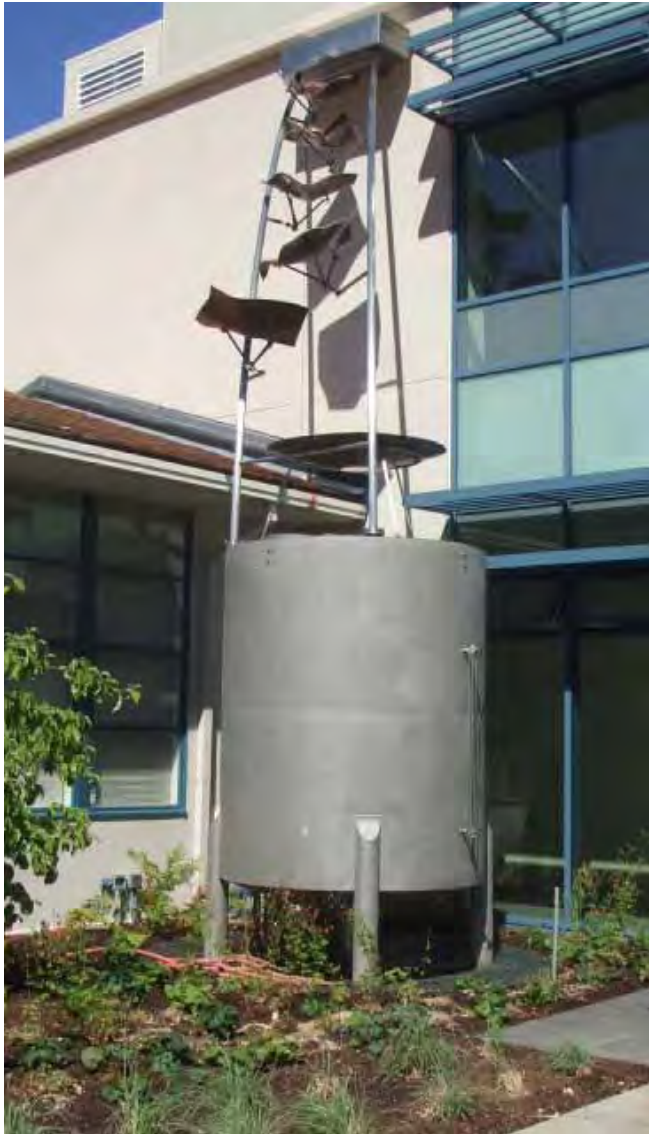
A cistern at Mills College in Oakland, CA is a stormwater BMP and a design element. Photo: Ingrid Severson
