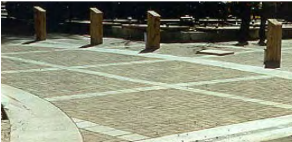
Permeable pavement can be integrated into a variety of hardscapes such as roads and sidewalks, plazas, terraces and patios.
