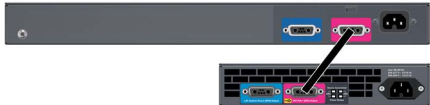
Figure 2-18. Connecting the 630 EPS to a switch
