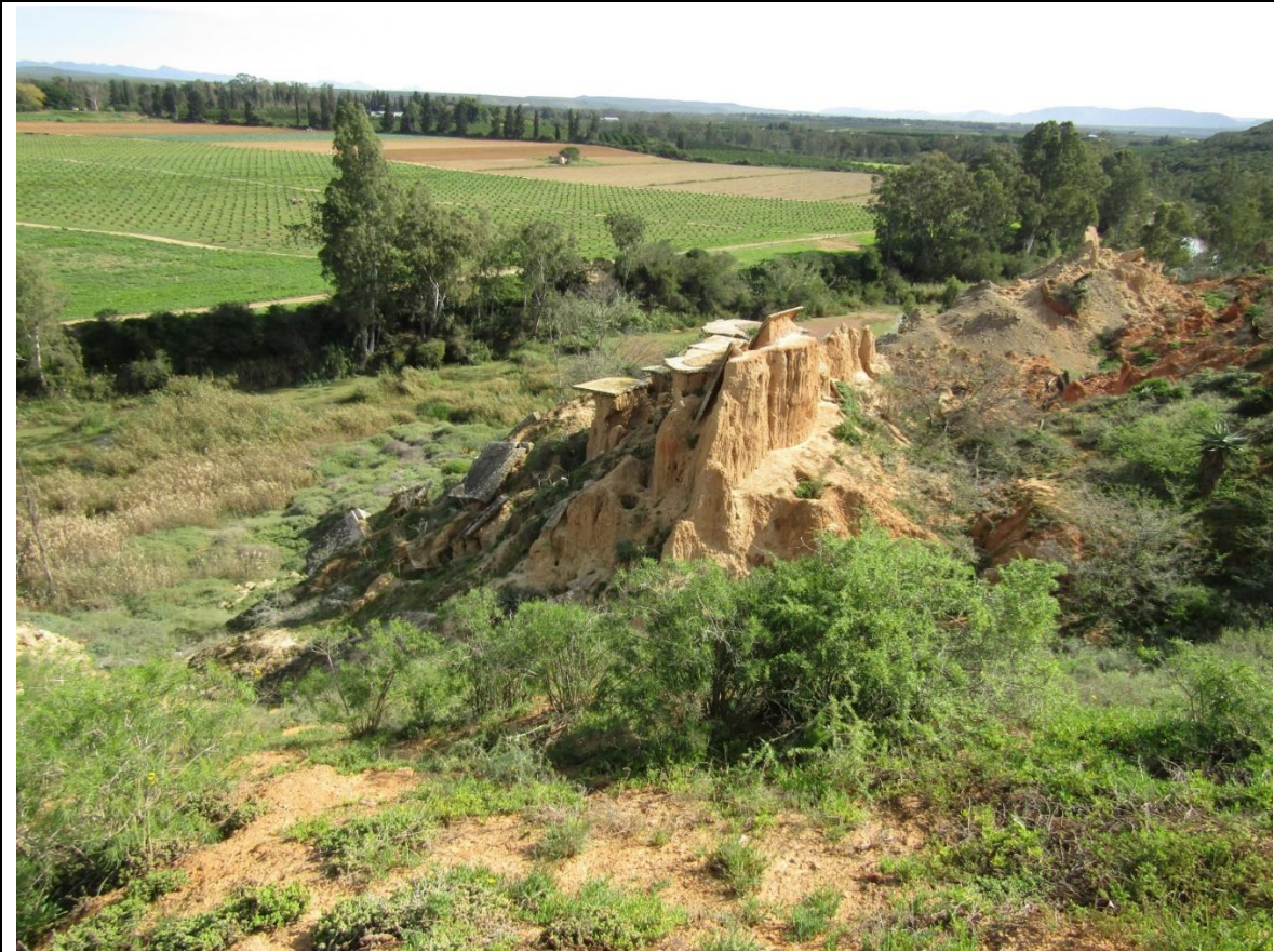
4.2. Erosion on the steep slopes at the north-western end of the property, also showing the defunct concrete canal that has broken mid-slope.
