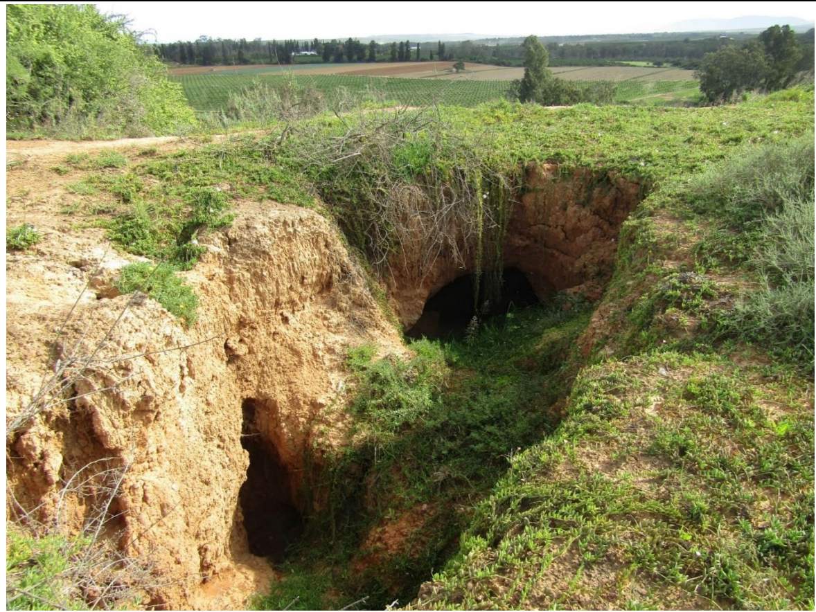
4.1. The 'erosion hole' or donga proximate to the proposed residential unit and the very steep slopes leading down to the Sundays River.
