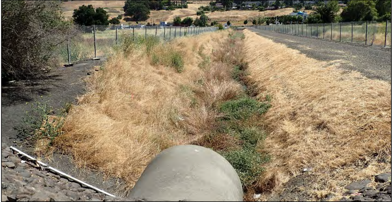
Photograph 1. The Alameda County Flood Control Channel location within the central portion of the Project Area. Photo taken from the culvert outlet at the southwest end of the channel. View facing northeast. Photograph taken June 15, 2017.
