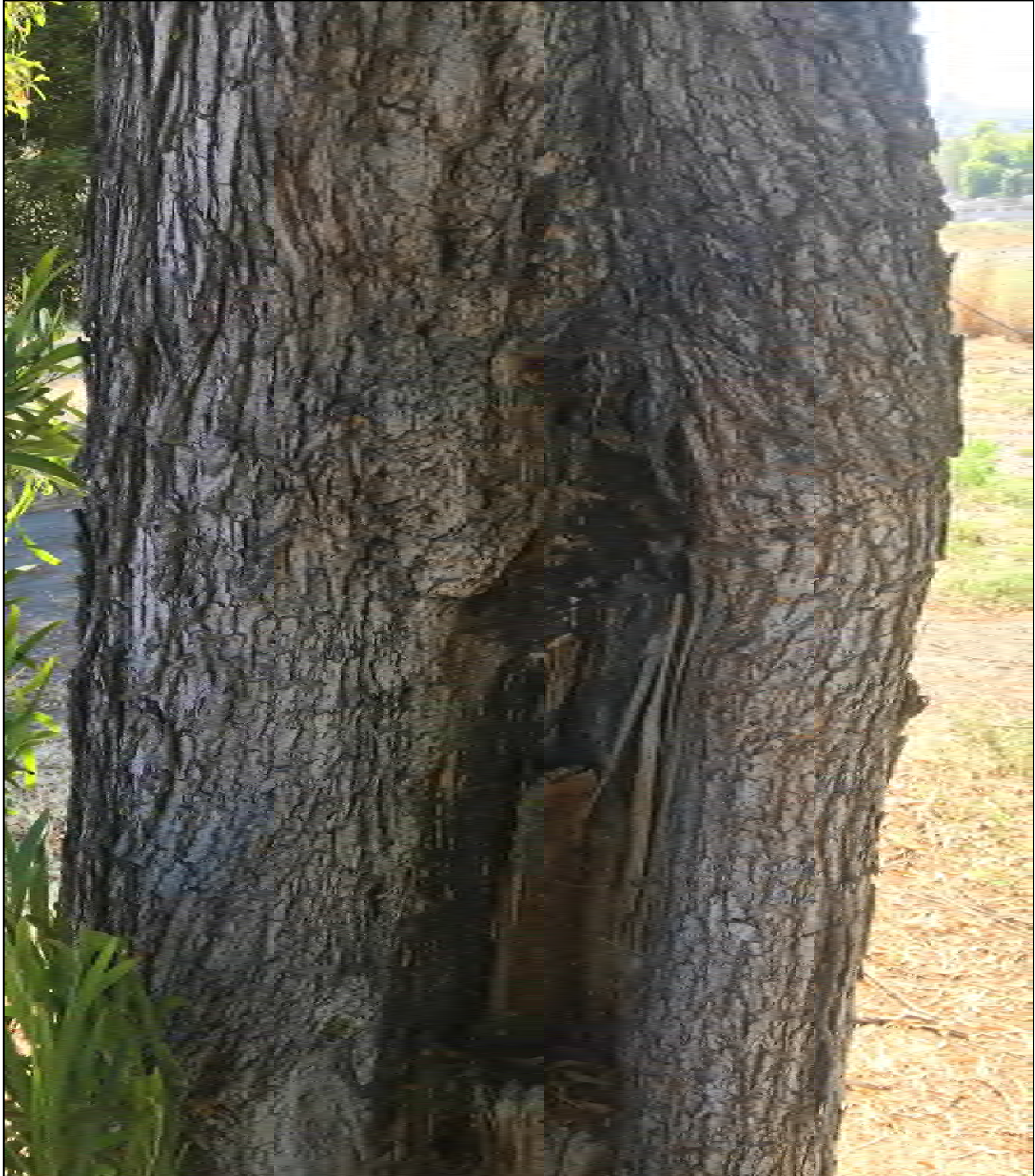
Photograph 5. Photograph depicting protected tree #587, a 22.1-inch DBH blackwood acacia. The major trunk cavity shown in the photograph was assessed as a significant structural defect. Despite the defect, the overall appraised value was determined to be $1,370.
