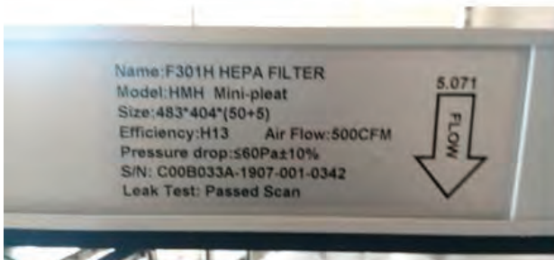
HEPA Filters (with blue pre-filters) installed over exhaust vent on Feb 11 2020
