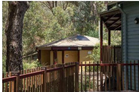
Figure 15. The toilet block viewed from the verandah to the rear of the building. (Source: Context 2020)
