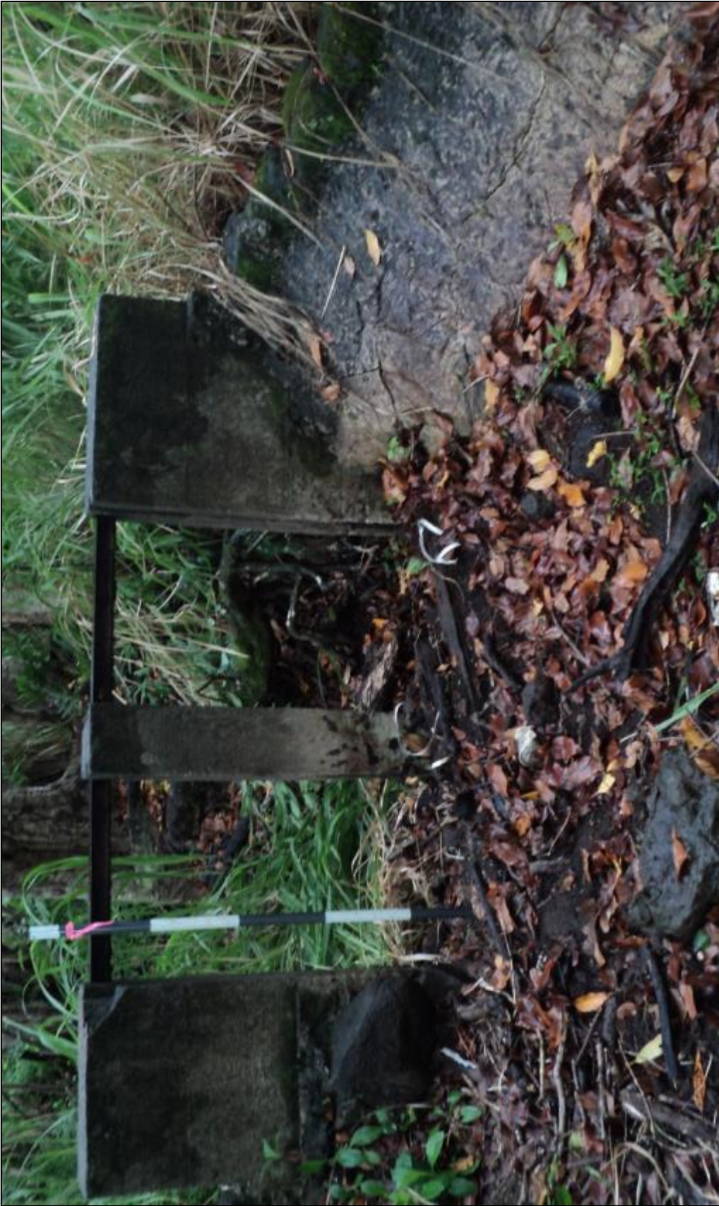
Figure 68. Site -2262 double gate with cement and rock wall to prevent erosion. View to north.
