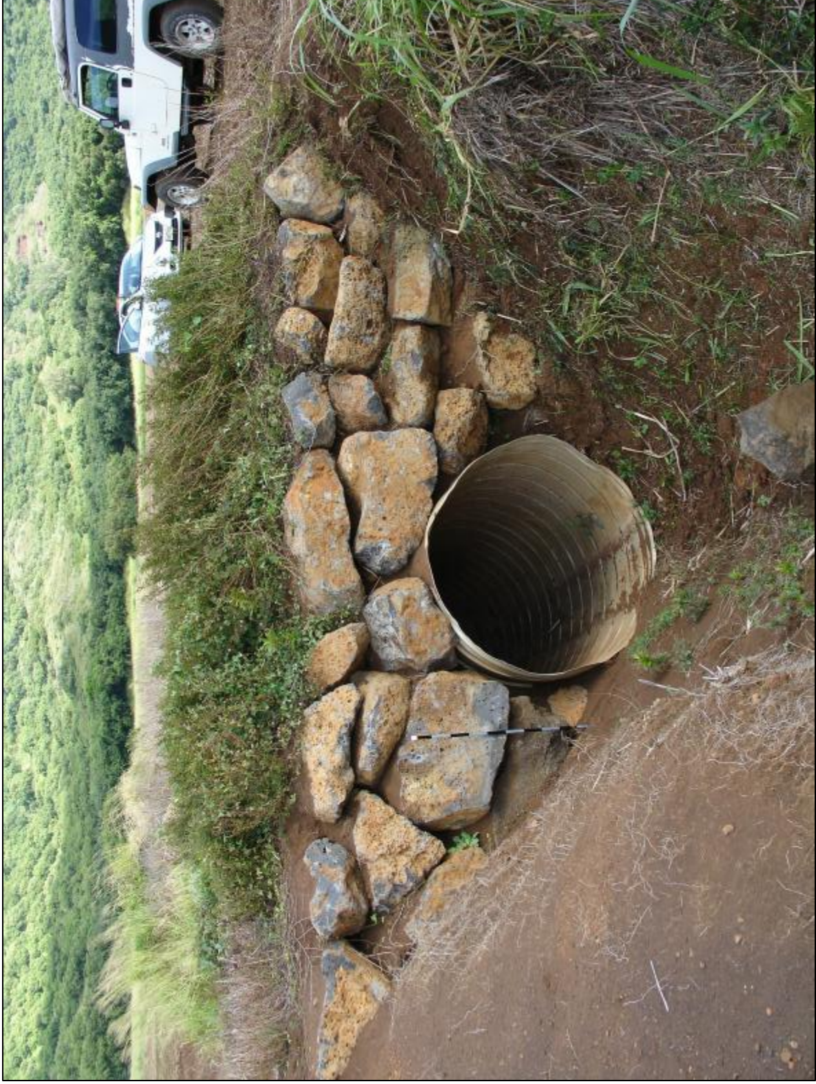
Figure 40. Site -2255, Feature 3 culvert. View to north. Representative example of all four culvert features rebuilt in 2014.
