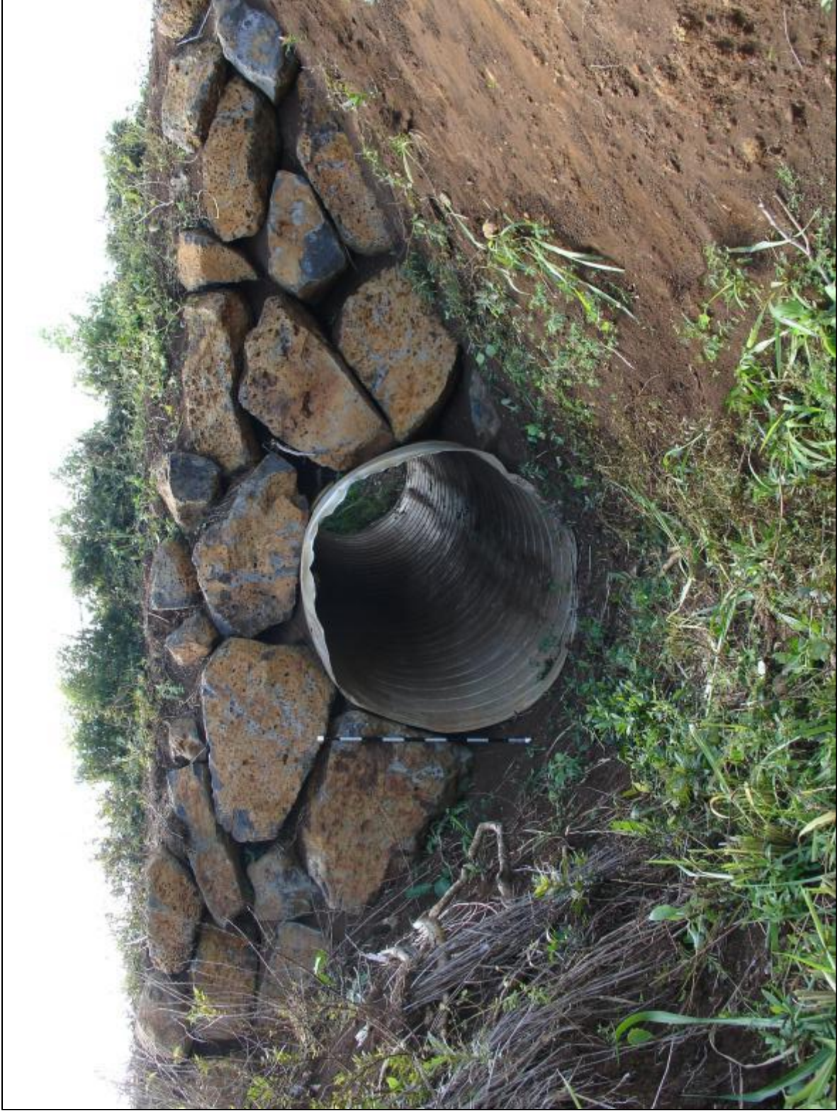
Figure 41. Site -2255 Feature 3 culvert. View to south. Representative example of all four culvert features rebuilt in 2014.
