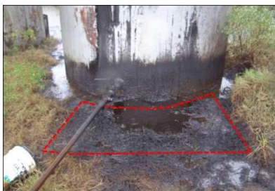
Figure C-13. Stained area under valve of large fuel tank designated as a small DU to document the presence of a release.
