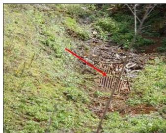
Figure C-14. Stormwater drainage vault designated as a DU for testing of sediment runoff from a contaminated property.
