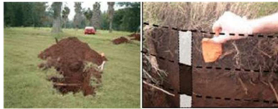
Figure C-10. Backhoe potholes used to collect increments from three subsurface layers designated for DUs at a former golf course (see Figure C-9).
