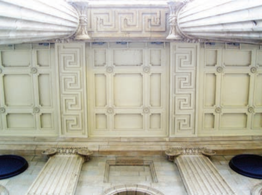
A view of the underside of the portico shows the Greek Key fret motif that recurs on the exterior and reconstructed interior of the GPO.
