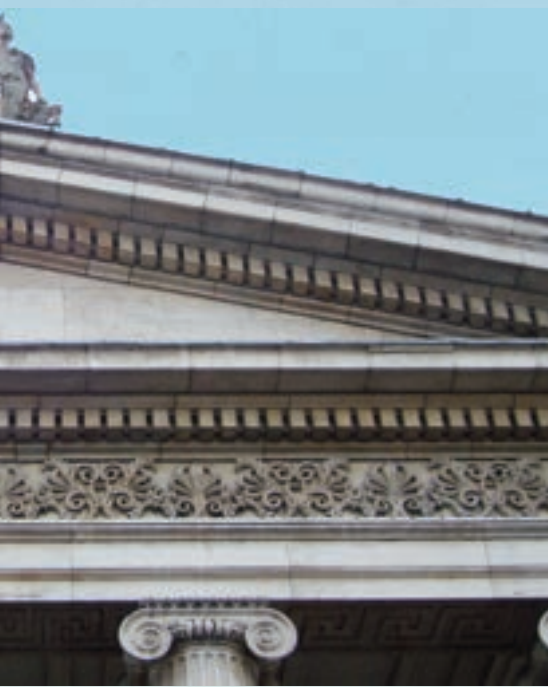
be over-painted with green, the Royal Coat of Arms, a feature of Portland stone insert, slightly brighter than the surrounding Portland stone at the GPO.
