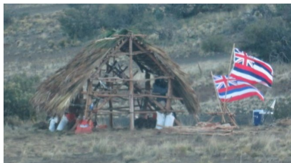
Figure 1: "Hale" in process of being built with 'ōhi'a wood and non-native palm fronds.
