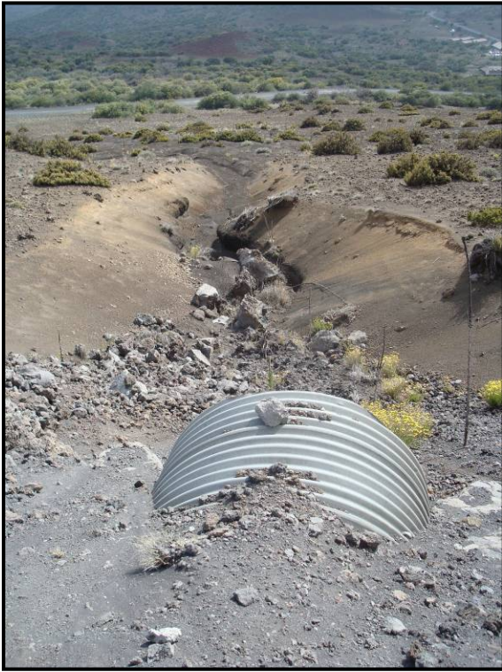
Figure 3-11. Mid Mountain Drainage Infrastructure
