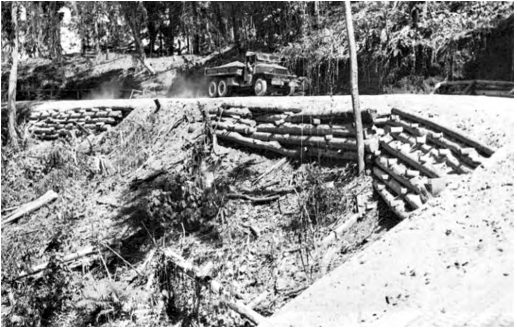
SUPPLY ROAD ON BOUGAINVILLE built by Army engineers. Note how coconut logs are used to support steep bank and underside of road.
