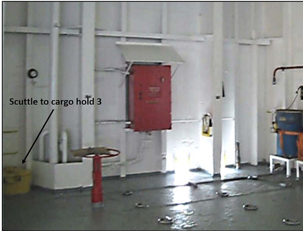
Figure 57. Second deck scuttle to hold 3. (Photo by former El Faro second mate)
