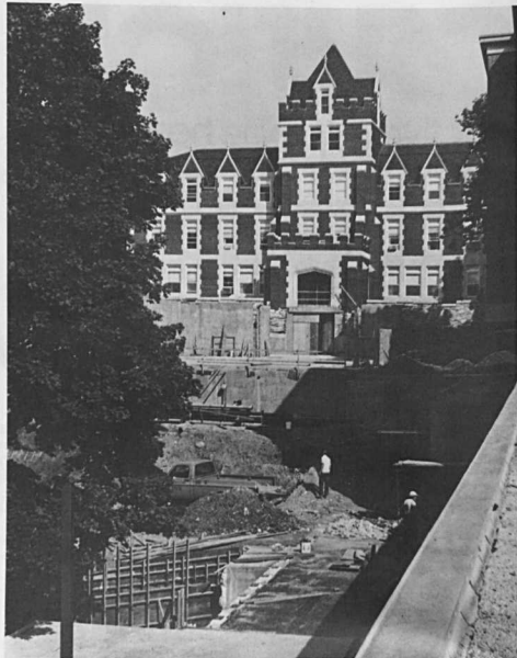
Elderidge Hall appears to be supervising the construction of the New Decker College Center, rising up at its feet. "We're working close to schedule with the completion date still set for June 1, 1978," reports Preston S. Yingling, director of the physical plant. The water line is completed and all utility lines have been placed in the new tunnel connecting with Elderidge. Steel was being set during the first week of July, allowing for the laying of the first floor.
