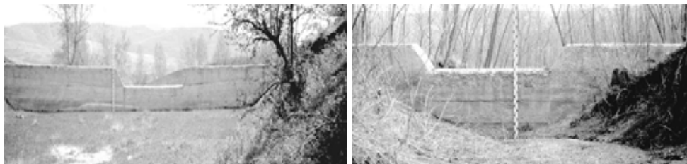
Figure 2. Checkdams on the gullies uncompletely siltated due to unsatisfactory correlation between the design of the checkdams and the versants' management
