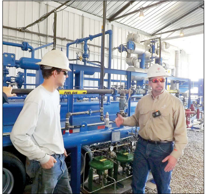
Russell Rankin, Statoil's Bakken regional manager in North Dakota, explains how this skid-mounted equipment strips out liquids before the gas is compressed into CNG. The last mile fueling solution is a partnership between GE, Statoil and Ferus. (Photo by Denis Smith)
