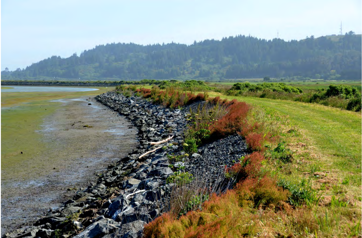
Figure 11. Hookton Slough on South Bay is an example of an earthen dike with rock revetment and roadway that is being maintained.
