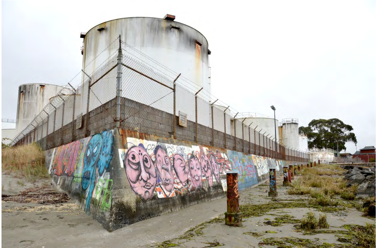
Figure 14. Eureka Bay is an example of a concrete bulwark forming the shoreline of Humboldt Bay.
