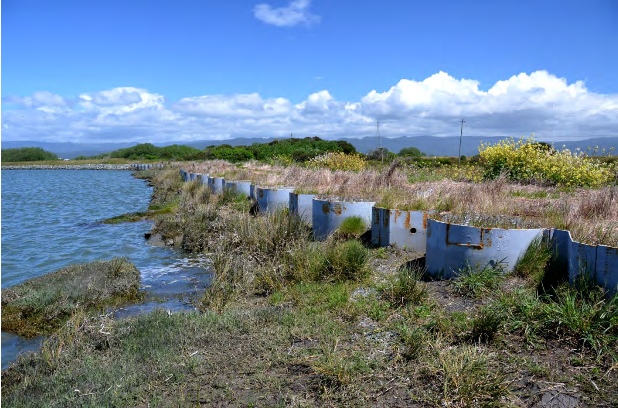
Figure 29. Mad River Slough is an example of a shoreline that is covered by a steel bulwark on Humboldt Bay.
