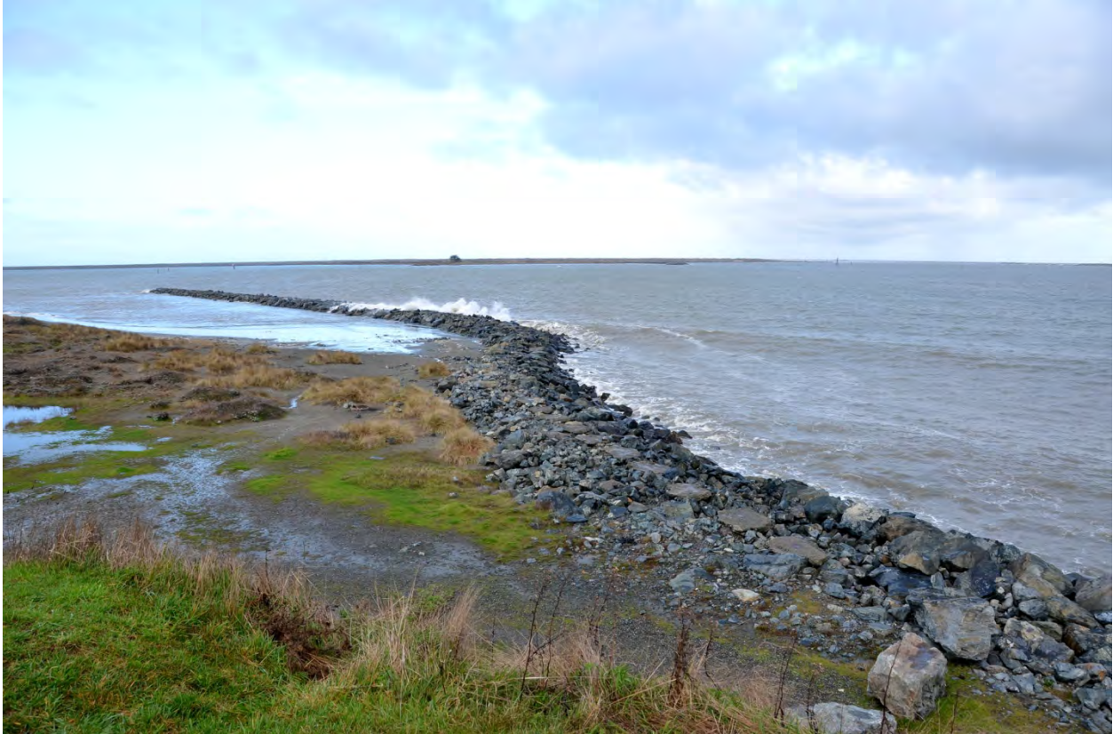
Figure 22. King Salmon on Eureka Bay is an example of a jetty forming the shoreline of Humboldt Bay.
