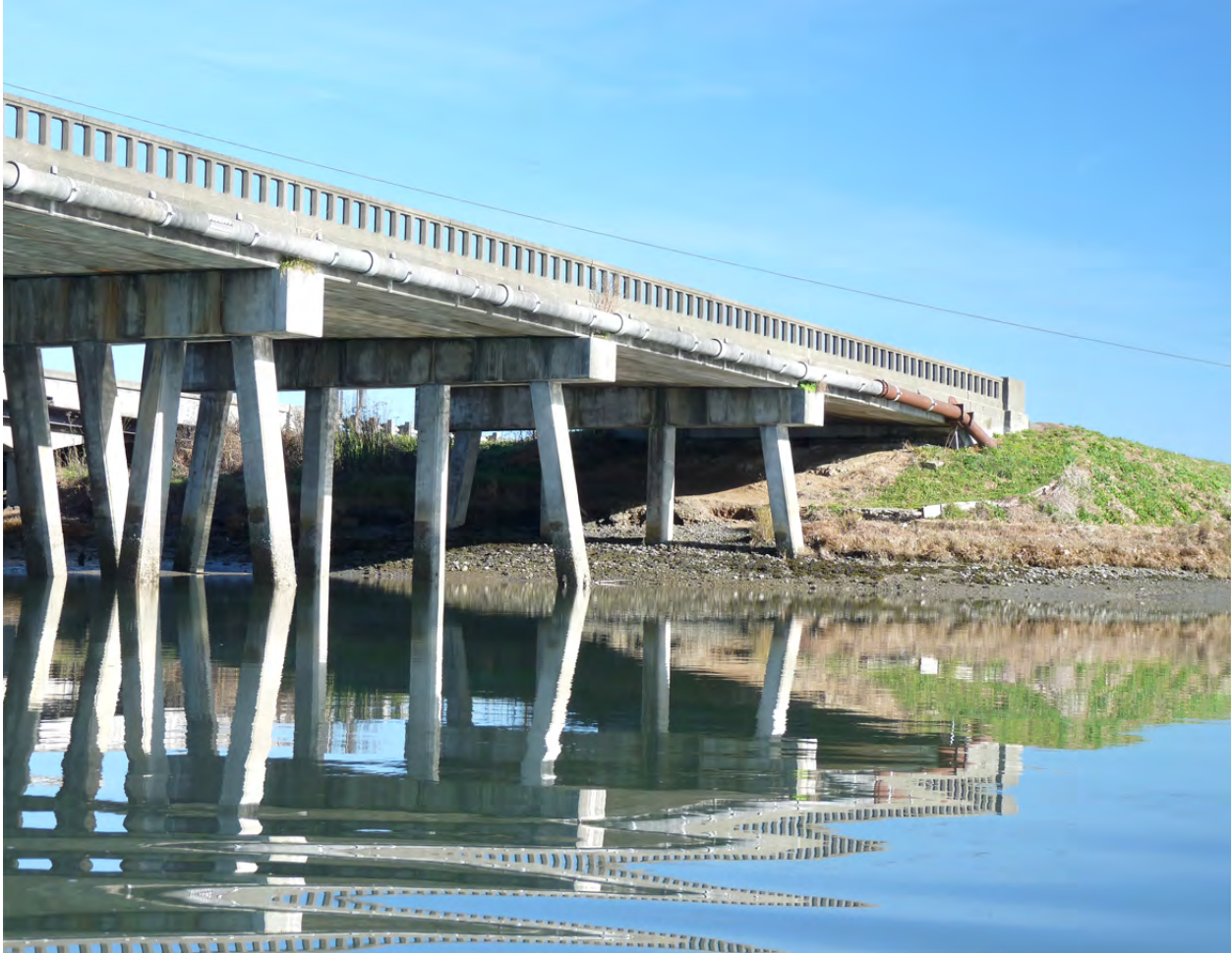
Figure 18. Eureka Slough is an example of a bridge abutment forming the shoreline of Humboldt Bay.
