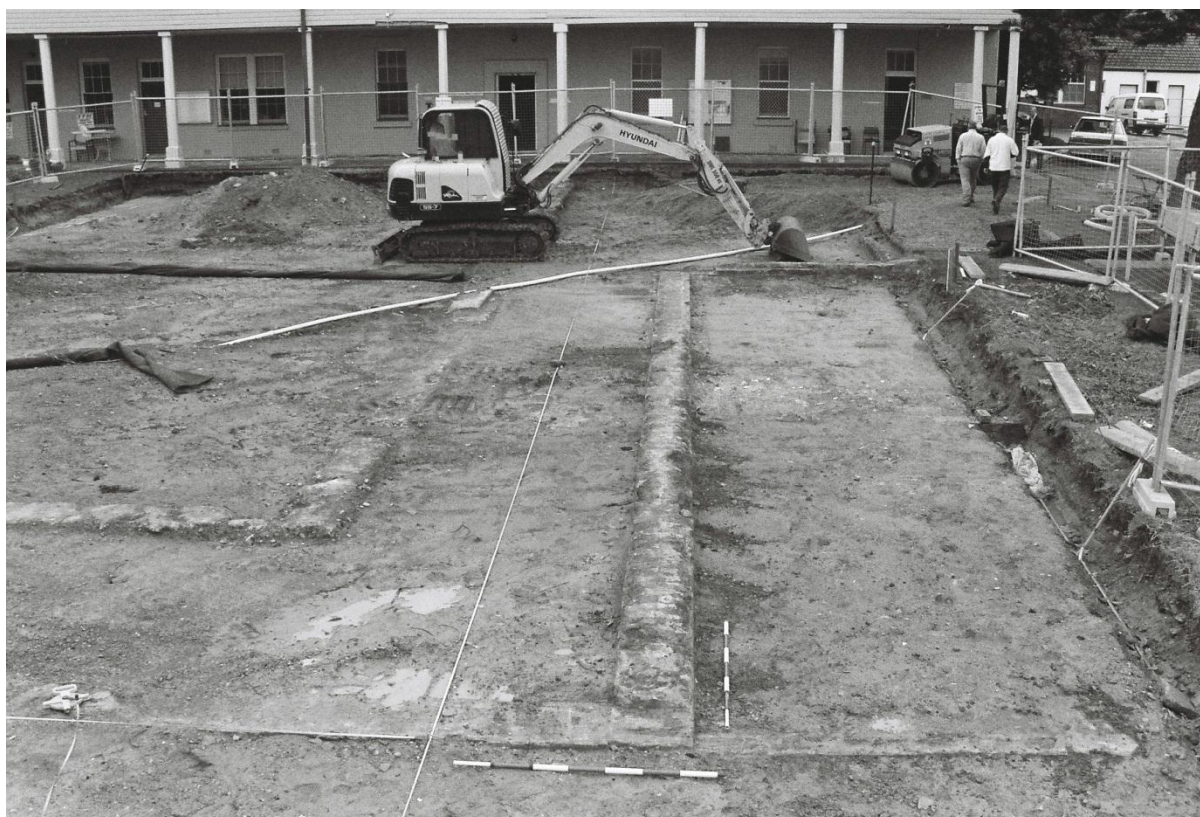
Figure 1.11 View of greater area of excavations. Note original barracks building in background. Facing west. (AMAC 2008: MWN8R110)
