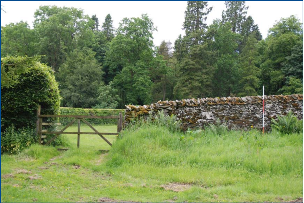
Plate 5: General view of the east wall to the south from the east
