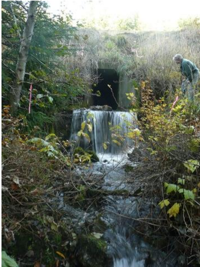
Telephone Creek Culvert south entrance with dropoff. (Photo: WTI)
