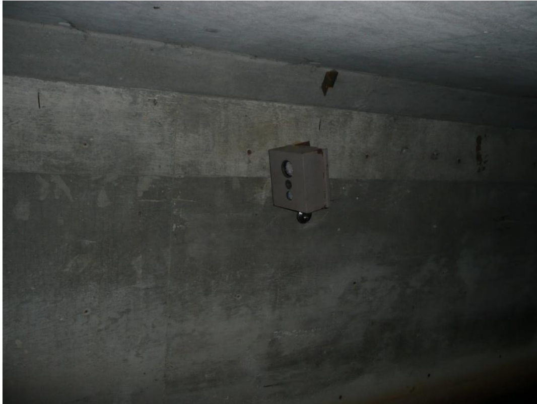
Figure 3.3. Remote camera deployed on culvert wall in a locked, metal security box. (Photo: R. Long/WTI)
