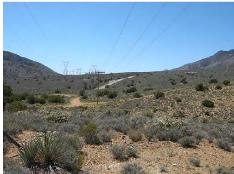
Photograph 8. Looking west towards the Mountain Pass Substation – black bush and juniper habitat.
