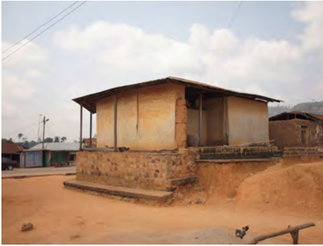
① The Spectators' Room at the back has collapsed.
