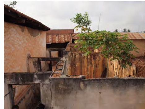
⑤ The four rooms that are part of the house complex have no roof.
