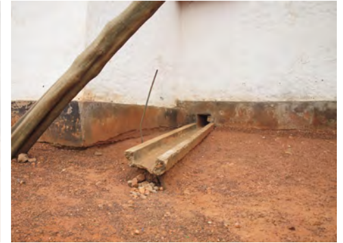
④ Noticeable erosion of the ground on the northern side.
