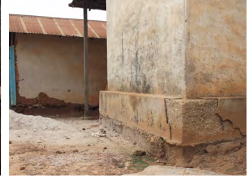
③ The ground at the back of the Shrine Room is highly eroded and over one foot of soil is missing due to erosion.
