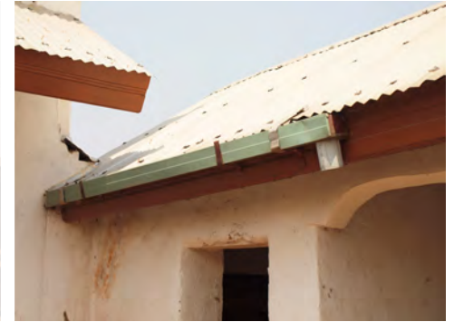
③ Unsightly roof gutter added to the northern corner of the courtyard.
