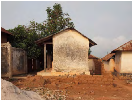
③ The mud wall hiding the mausoleum building has collapsed.
