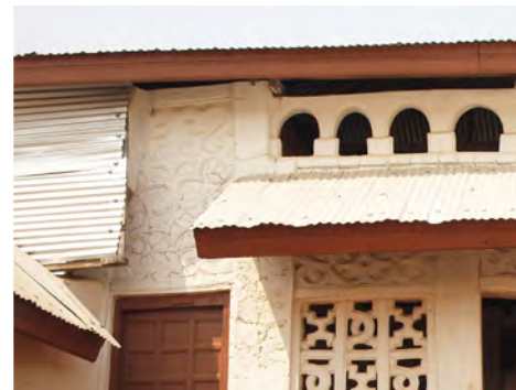
⑥ Another unsightly temporary protection has been added to the Shrine Room (located to the left of the temporary roof).
