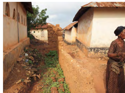
④ As a result, wall remains are blocking water drainage.
