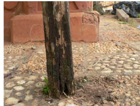
⑥ Wooden poles supporting the roof are rotten at the base.
