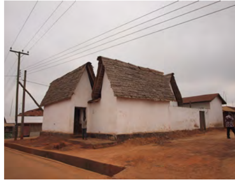
② The traditional roof restored in 1999 is still in place, the raffia shingles have been replaced 3 times.
