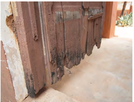
④ Many wood elements, including shutters, doors, and roof elements, are rotten or affected by termites.
