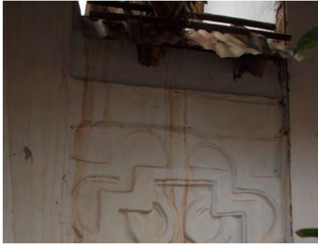
① Some roof elements are leaking.
