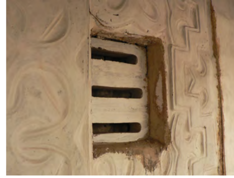
② One of the wooden shutters has been replaced by cement blocks.
