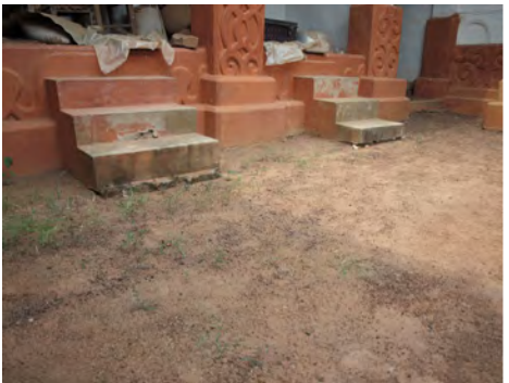
④ Some drainage problems exist in the courtyard along the Drummers' Room.
