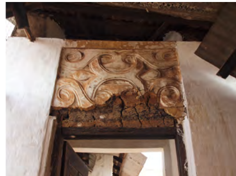
⑤ Decorative elements partially broken above the entrance.
