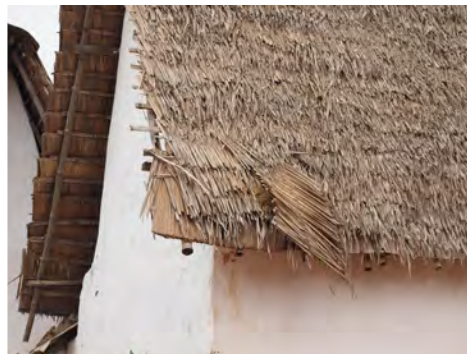
⑥ Some raffia shingles need to be replaced.
