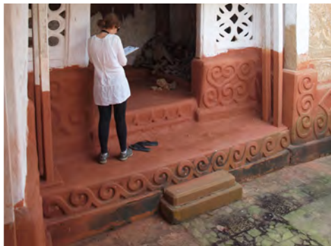
⑤ As a result, the red plinth is very humid.
