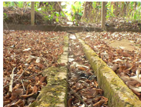
⑦ Gutters draining the site are currently blocked but they can easily be cleaned.
