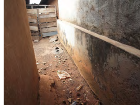
② Corridor on the southern side is very narrow and water evacuation is difficult here.
