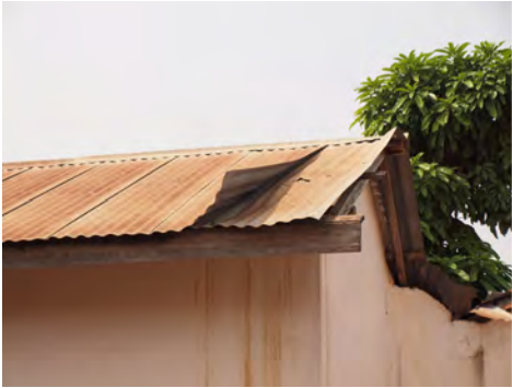
① The roof requires attention as it is leaking.
