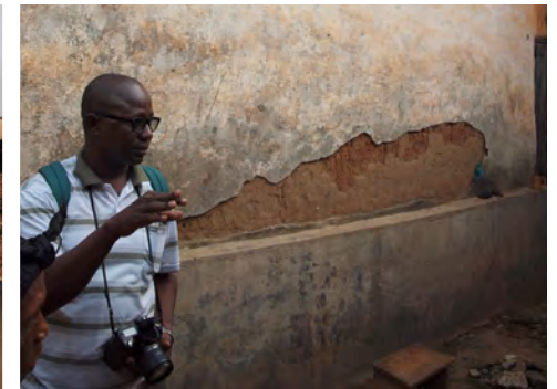
⑥ The sand-cement screed on the external walls contains a great deal of damage and many parts have started to peel off.
