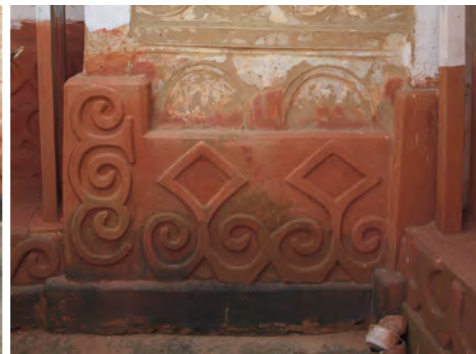
⑥ Also, the red base around the courtyard is very humid and covered with moss in some places.
