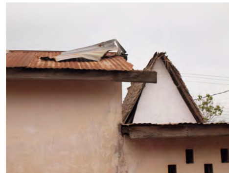
⑦ The adjoining house is leaking. One of the roofing sheets is already torn.
