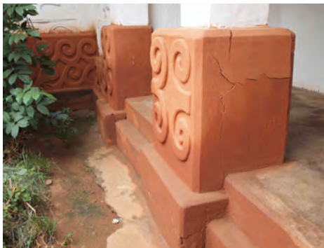
⑤ The high humidity level is affecting decorative elements and there are cracks in the cement plaster at plinth level.
