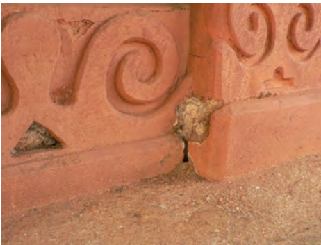
④ Termite holes can be seen at the base of the walls.
