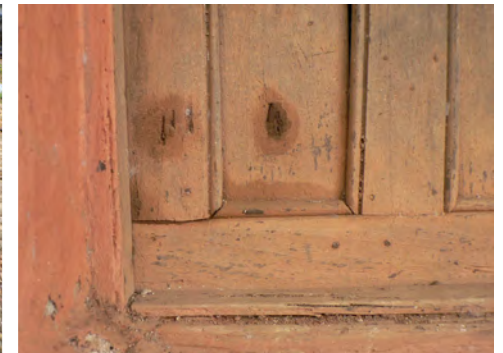
⑦ Termite infestation is affecting all of the wood elements.
