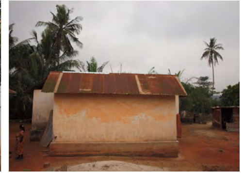
④ GMMB conducted repairs on the roof above the Drummers' Room in 2013.
