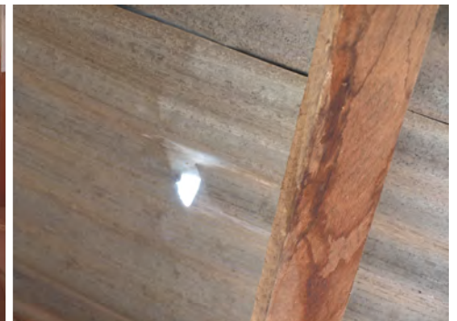
⑦ Roofing sheets contain holes.
