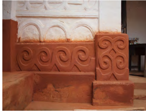
② Humidity is very high in the wall base due to the dome-shaped courtyard.
