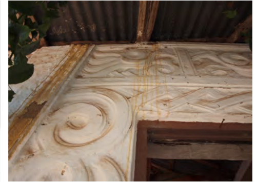
③ Water is dripping on the decorative elements in several places and slight erosion has already occurred.
