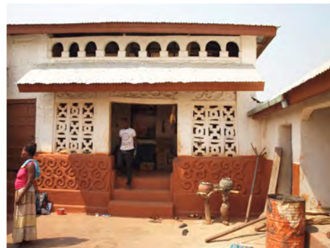
⑤ The temporary roof installed above the decorative elements in 1998 to protect them from the rain is conspicuous but working well.
