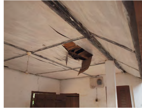
② Ceiling boards in the adjacent house are damaged by humidity.
