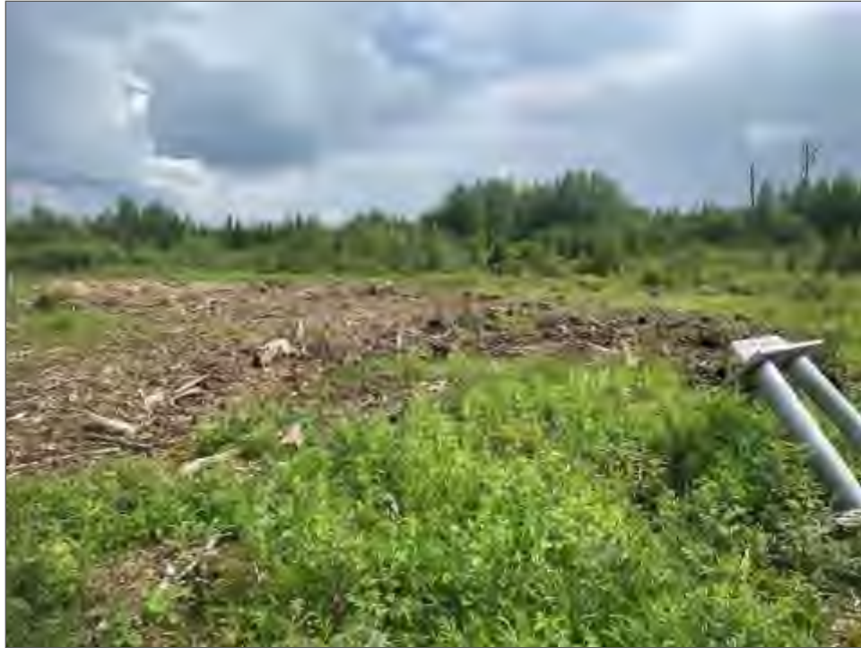
Plate 3.3-11. Modified (clearing and tower construction) on the edge of the Wm01 Beaked sedge - Water sedge marsh at Plot PI2.
