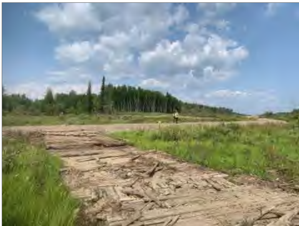
Plate 3.3-8. Construction road and rig mats bisecting a Wf02 Scrub birch- water sedge fen at Plot MWL02.
