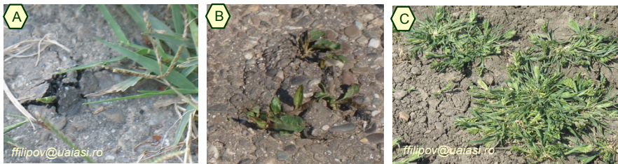
Fig.1 Degradation of asphalt alleys after growth of Cynodon dactylon (A) and Convolvulus arvensis (B). Sclerochloa dura (C) as bioindicator of extremely superficial strong compacted soils
