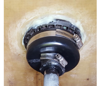
Example of Blueline Small KFD Repaired
