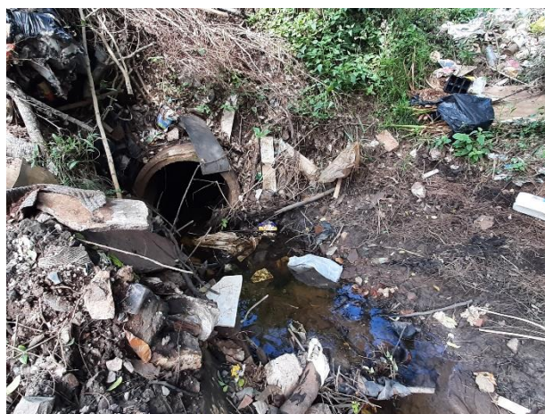
Photo 5: View of the culvert at the toe of the wetland. The culvert conveys outflow from the wetland into the Msimbazi Estuary.
