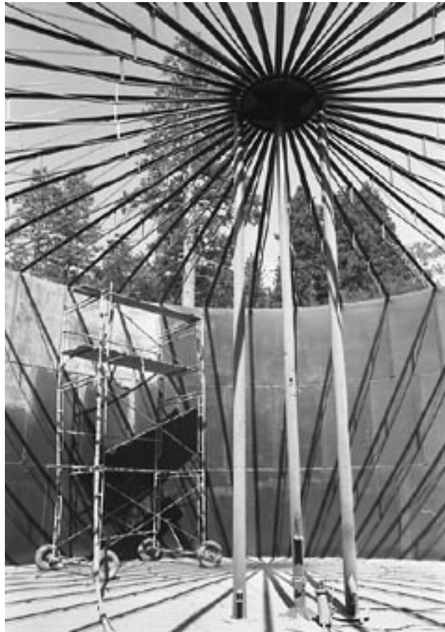
This unusual view of the inside of one of Fern Valley Water District's storage tanks was made possible in early September 1986 when the tank was partially disassembled for repairs. The 24-foot, 420,000-gallon tank near Humber Park was one of two at the site repaired that summer.
