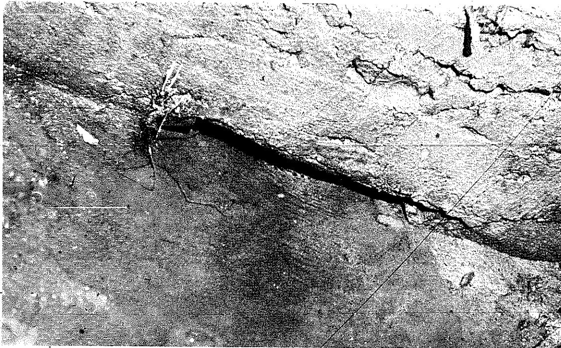
PLATE 321 Point D, view of water coming under a small partition as it goes through the trough.
