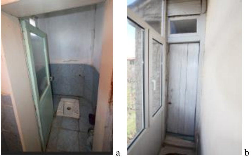
Figure 15. Room-ZK-03(a) toilet area and Room-1K-01(b) toilet balcony of registered house on Block 137, Parcel 32 (From author's archive, 2018)
