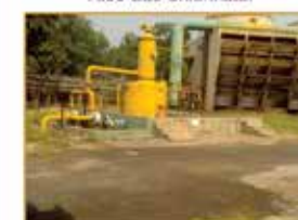
Chlorine Leak Absorption System
