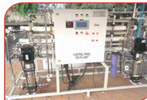
Reverse Osmosis System
