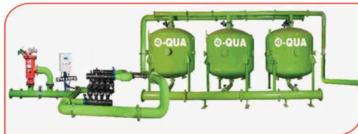
Fully Automatic Water Filtration system
