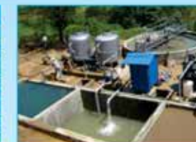
EFFLUENT TREATMENT PLANT CHEMICALS
