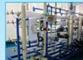
RO MEMBRANE TREATMENT CHEMICALS
