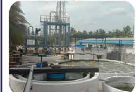
200KLD ZLD Plant
