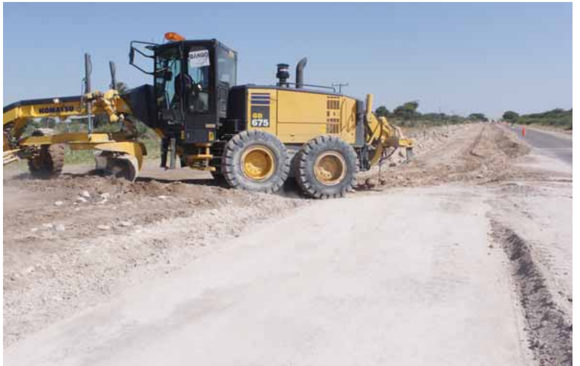
Gumare-Sepopa road maintenance major works have started with shoulder widening as the first step. Mr Moichubedi said the project, which was awarded to Bango Trading Company for the 70km Gumare-Sepopa section at a cost of over P343 million was expected to take 18 months. Photo: Kedirebofe Pelontle
