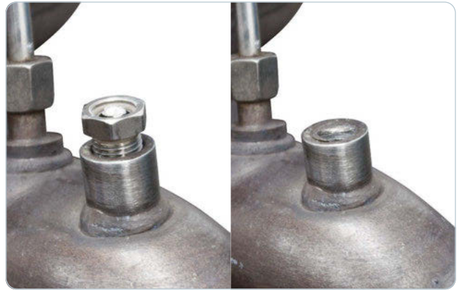
2. Left: After removal of sensor line Right: Temperature sensor removed; Threading damaged
