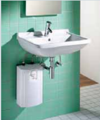
Large storage tanks spoil the appearance of the wash place and needlessly consume a large amount of energy
