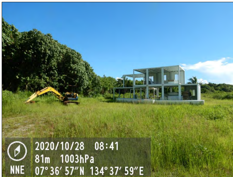
Figure 21. Framed structure being built on old crusher plant area in the south-central half of SD 2. Image taken on current access road facing north-northeast. See Figure 23 for location of structure.
