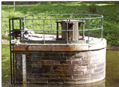
DG26: Monikie Reservoir: this in situ sluice regulates levels between the north and south basins.
