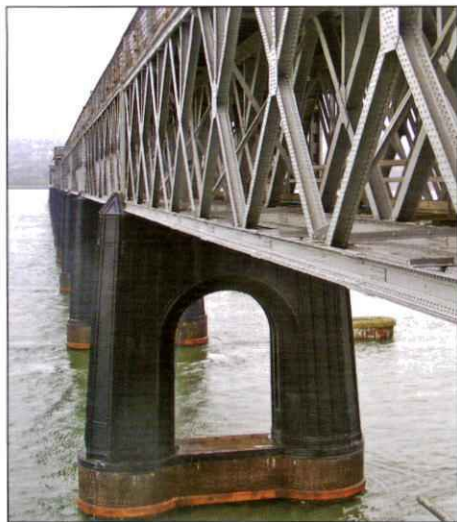
DW15: Close-up view of a pier on the Tay railway bridge from near the middle; on the right, one of the remaining bases of the original piers
