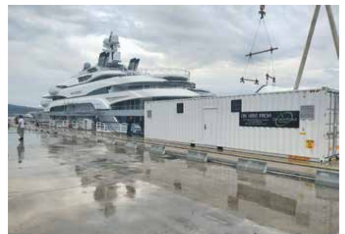
High Power Shore to Ship Solution
