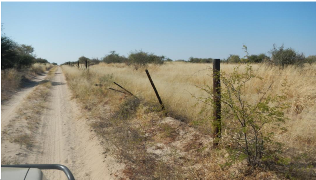
Plate 10 Elephant damage along the Kuke Fence
