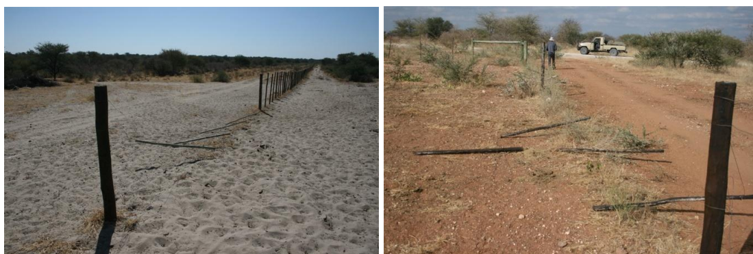
Plate 16 The Hainaveld protection fence, damaged in places allowing the free movement of livestock and wildlife between Hainaveld west and the Lake Ngami area
