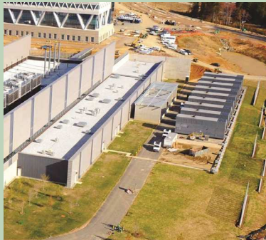
Detached Central Utility Plant (CUP): 72 Hour Back-up Power + Redundant Utility Feeds
