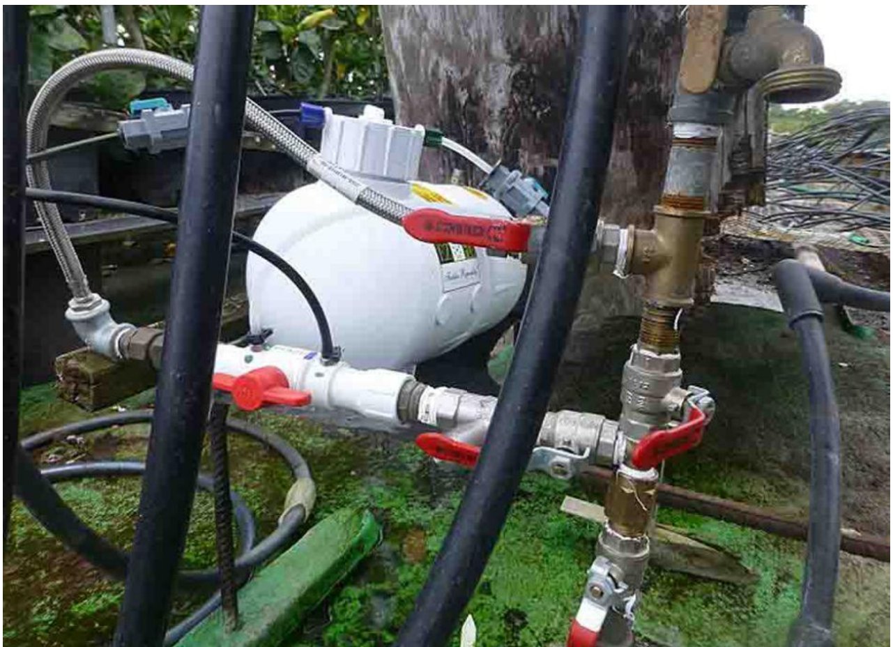
Below: The valve system modification to install the EZ Flow system. Looks complicated but in reality is fairly simple. On each side of the red "T" valve is the feed line to the tank "black' and the fertilized return line 'clear"- hard to see in photo.
