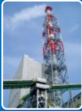
Tomakomai Mill's RPF boiler
