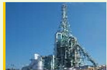
Oita Mill's RPF boiler
